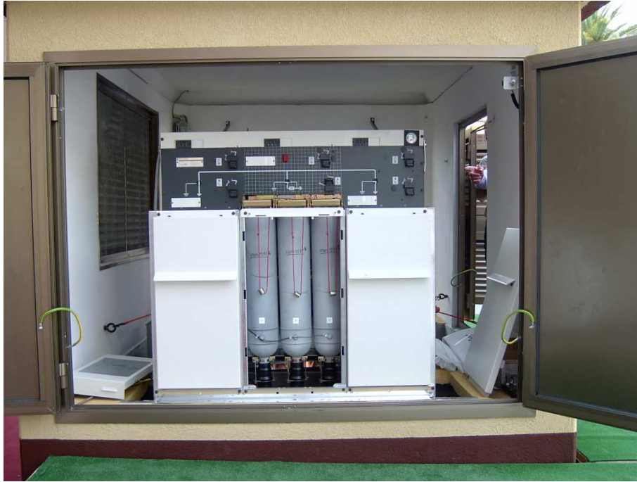
Figure 1. Typical Ring Main Unit in an automated TS MV/LV.
