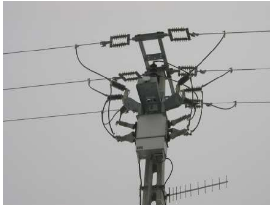
Fig. 3 Automated switch on the concrete pole
